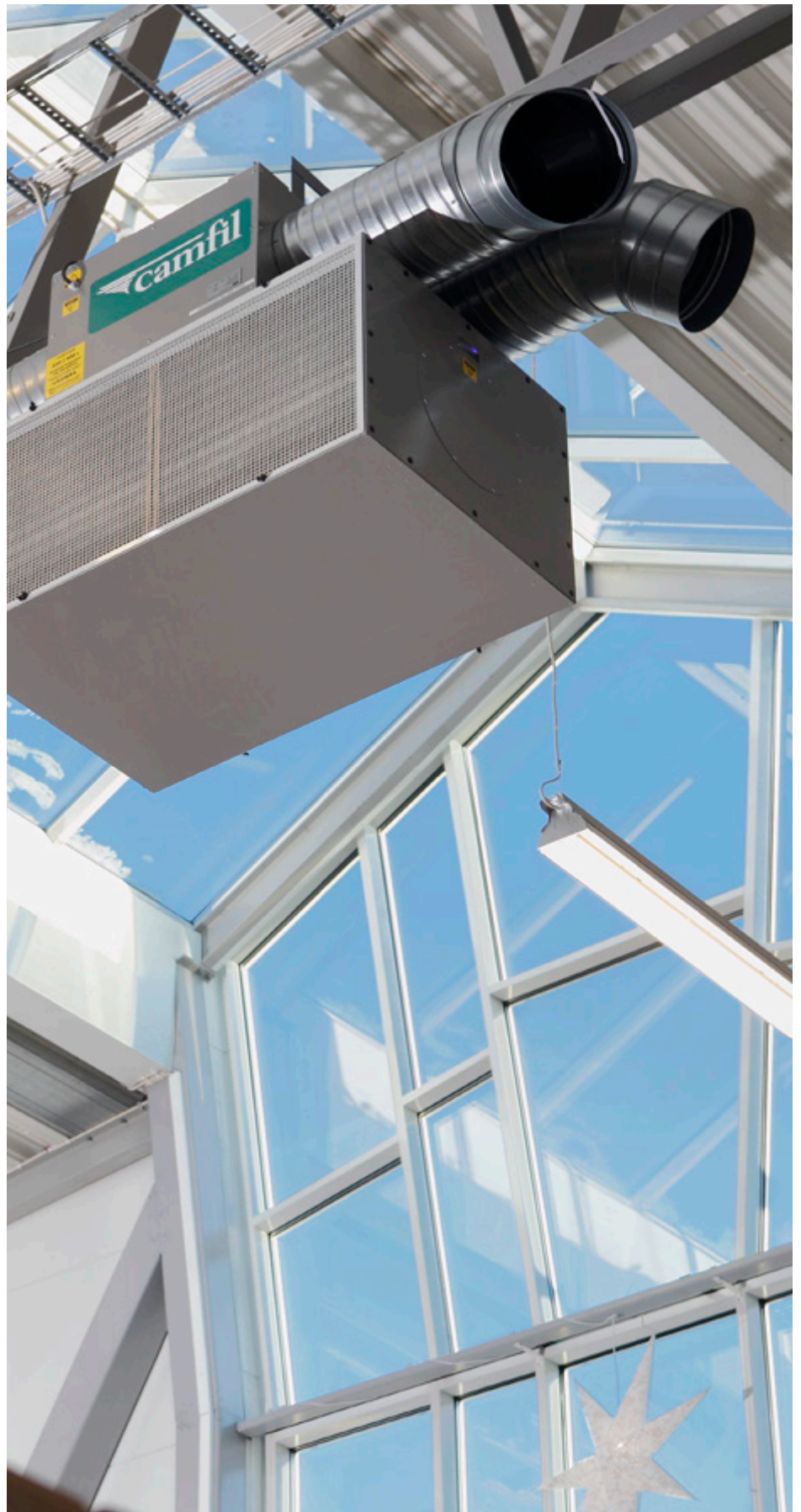
A ceiling-mounted air purifier efficiently purifies the air of nanoparticles as well as of large visible bits of dust. At the same time, the air is remixed, which provides a higher average temperature at floor level.
